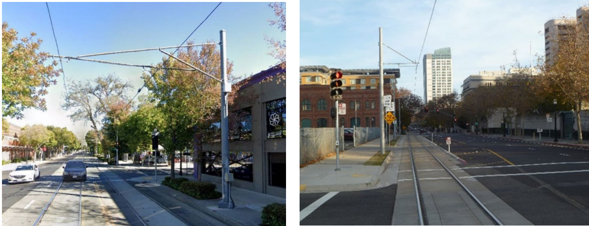
Figure 9 Photographs of Overhead Contact System
